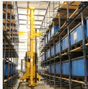
Automated Storage and Retrieval Systems
