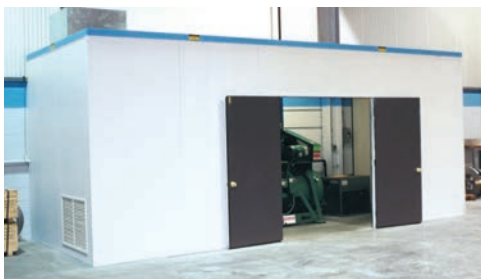
Unfinished compressor enclosure field painted to match plant color scheme.
